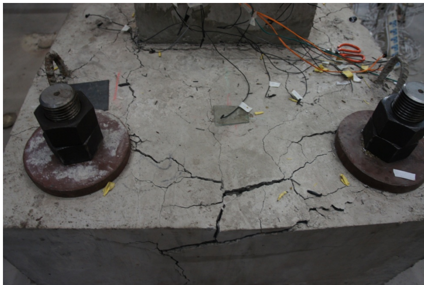
Fig. 8.13 Column Foundation Failure
