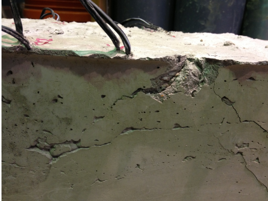
Fig. 7.15 Crack at Loading Point
